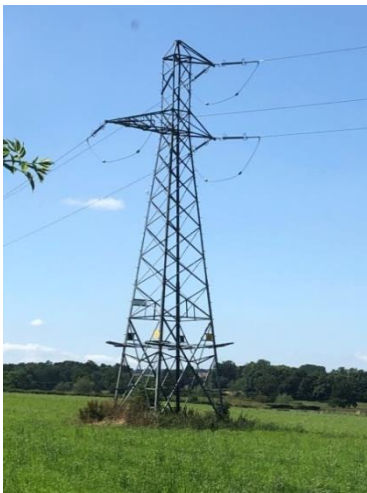
Figure 7 66kV Tower Mounted Overhead Power Lines
