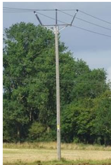
Figure 10 132kV Pole Mounted Triton Overhead Power Lines
