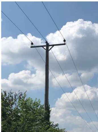
Figure 4 11kV Overhead Power Lines
