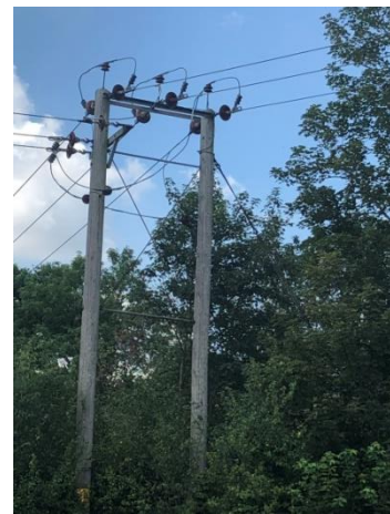
Figure 5 11kV Overhead Power Lines
