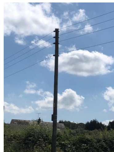
Figure 2 Uninsulated Conductor Low Voltage Overhead Power Lines
