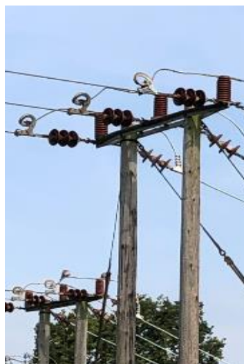
Figure 6 33kV Overhead Power Lines
