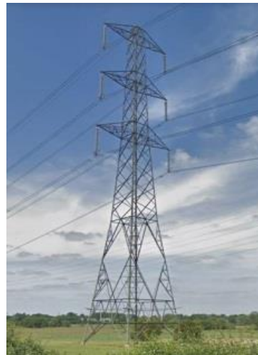
Figure 8 275kV - 400kV Tower Mounted Overhead Power Lines
