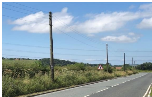
Figure 3 Three Phase, Neutral, Uninsulated Conductor Low Voltage Overhead Power Lines
